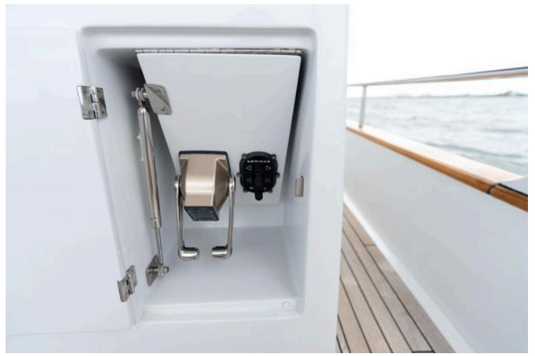
Aft deck controls
